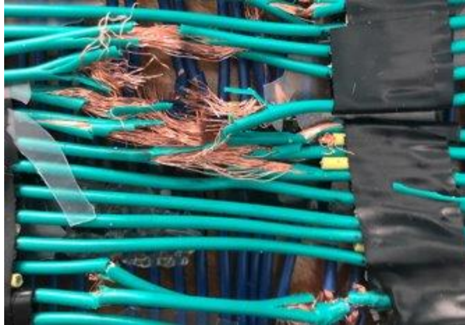
Figure 4-7: Wire Grid Breakage
