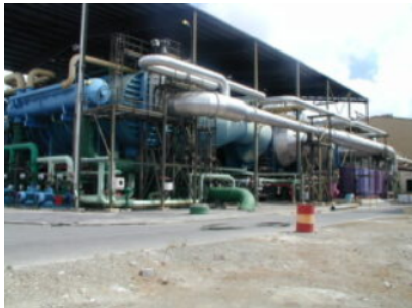
Figure 6. CaribDA Desalination Plant (CaribDA, n.d.).
