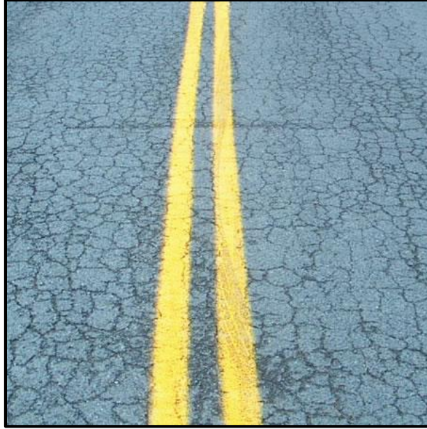
Figure 3 Cracking on road
