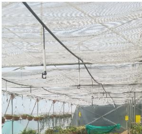
Figure 8: Foggers installed in a greenhouse
