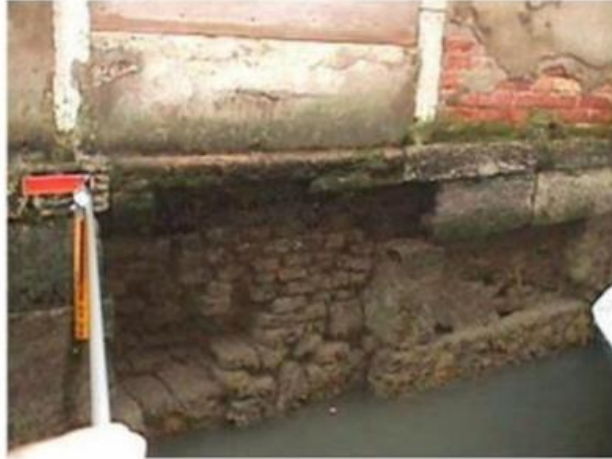
Figure 19: Canal Wall Damaged by Erosion
