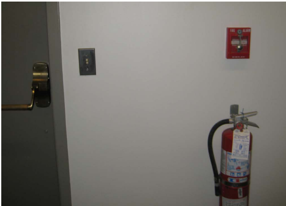
Figure 93: Pull station correct height and distinguishable (items 21 and 22)
