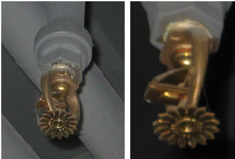
Figure 60: Sprinklers that need to be cleaned
