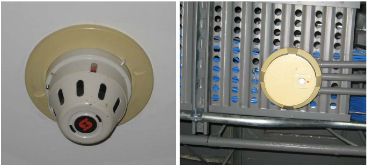
Figure 91: Marked Smoke Detectors (items 18 and 23)
