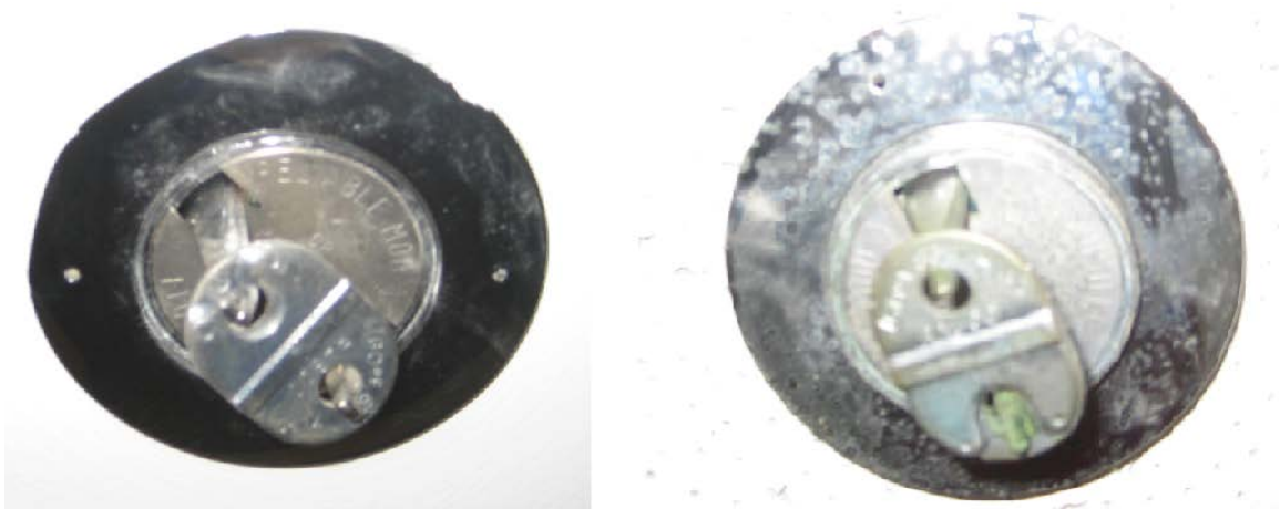
Figure 62: Fusible link askew on left sprinkler compared to right
