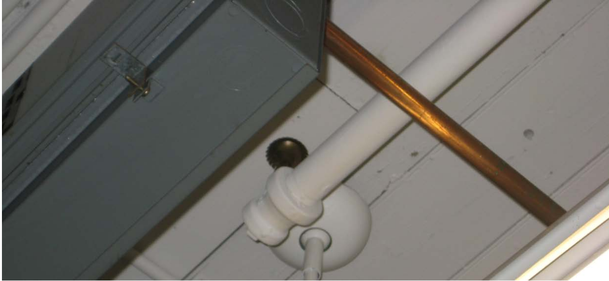
Figure 58: Metal Box Obstruction Room 107
