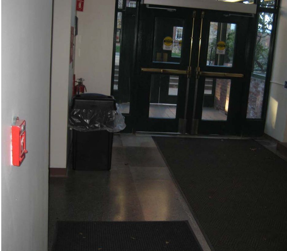
Figure 92: Pull station more than 5 ft from entrance (item 21)
