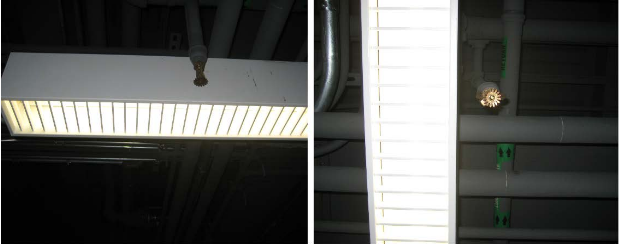
Figure 57: Light Fixture Obstruction Second Floor Hallway
