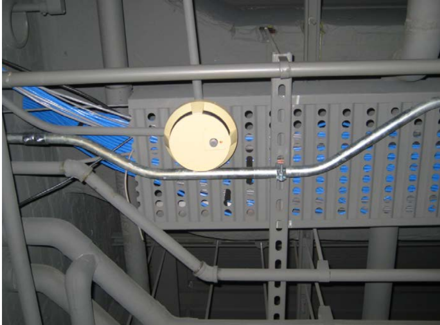
Figure 90: Smoke detector mounted and not recessed (item 14)
