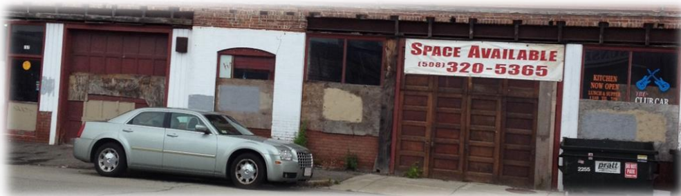
Figure 16: Blighted Building on Harding Street (Photo taken 11/1/14)
