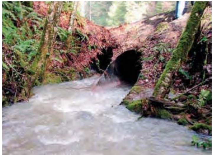
Angle measured from upstream channel to centerline of culvert barrel is from 15-45 degrees. 1
