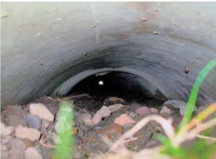
Blockage occupies 30-75% of opening. 1
