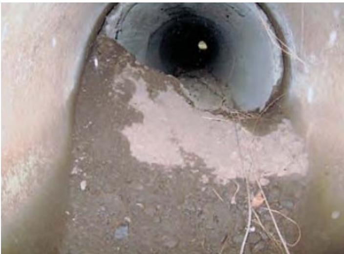
Significant separation of joints and seams between 1" to 3"; infiltration of backfill into culvert; voids visible in fill through offset of joints. 1
