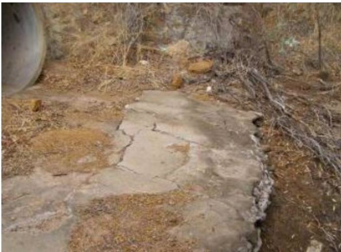
Significant cracking affects >50% of apron. Significant piping or undermining. 4
