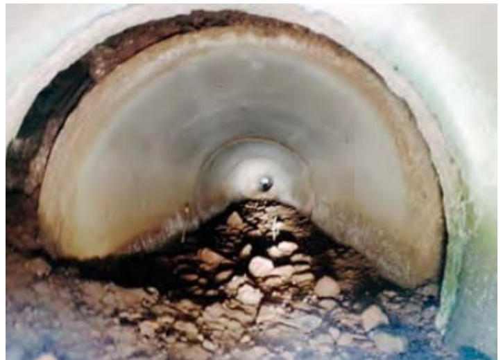
Severe separation of joints and seams greater than 3"; infiltration of backfill into culvert; large voids visible in fill through offset of joints. 1
