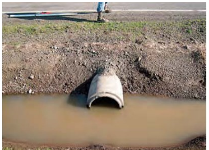
Angle measures from upstream channel to centerline of culvert barrel is larger than 75 degrees. 1
