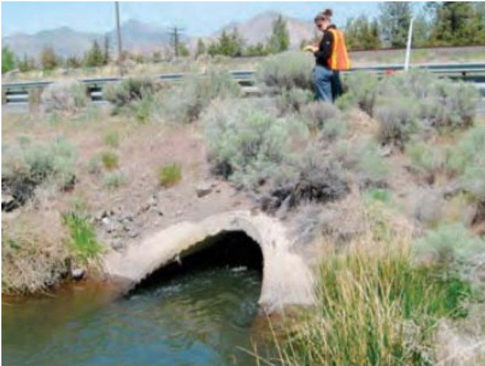
Angle measured from upstream channel to centerline of culvert barrel is from 0-15 degrees. 1
