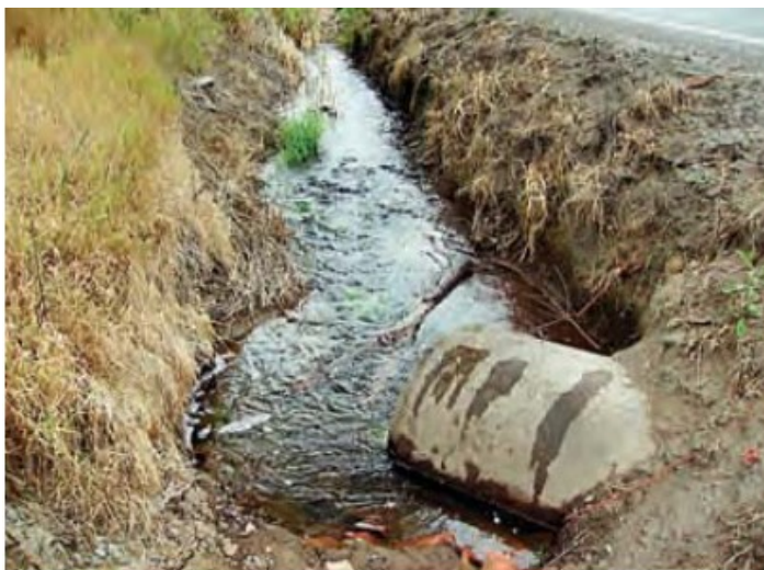
Angle measured from upstream channel to centerline of culvert barrel is from 45-75 degrees. 1
