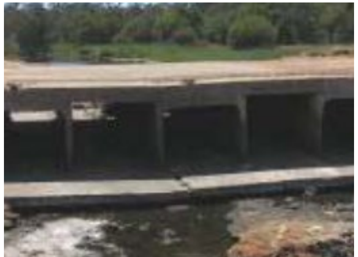
Partially or totally collapsed, significantly effecting performance and/or causing embankment and/or roadway damage. 4
