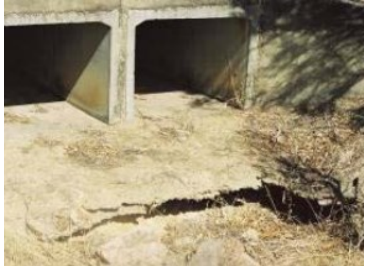
Minor cracking but no visible piping or undermining. 4
