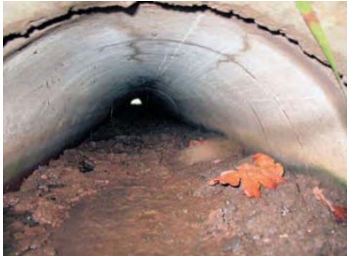
Blockage occupies 10-30% of opening. 1
