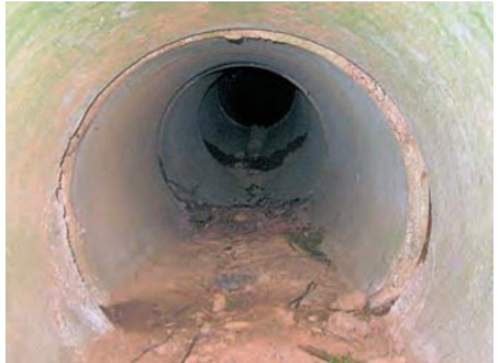
Minor separation of joints and seams up to 1", minor backfill infiltration. 1
