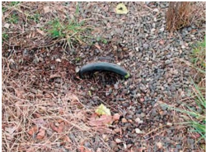
Blockage occupies >75% of opening. 1
