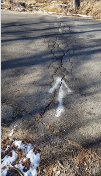
NOTE ROAD CONDITION
