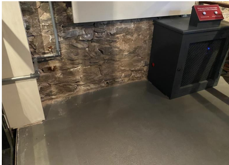
Figure 40: Damaged wall adjacent to elevator door in Candle Factory (S. Turner).
