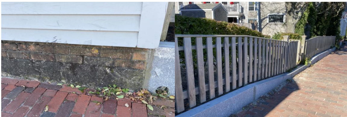
Figure 47: Floodwater damage on the foundation of the Discovery Center (left) and dip in block wall rear yard (right) (S. Turner).
