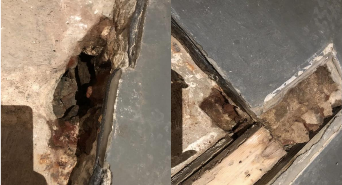
Figure 41: Close-up of breaches in foundation behind current elevator shaft (E. Rudd)
