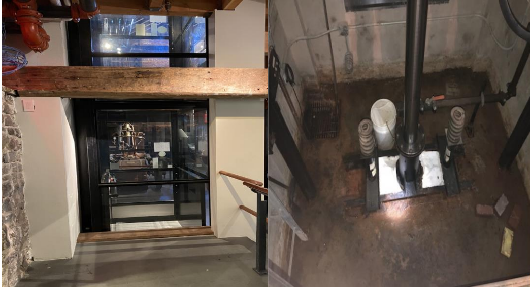
Figure 39: Side view of elevator (Left: S. Turner) and base of elevator shaft (Right: E. Rudd).
