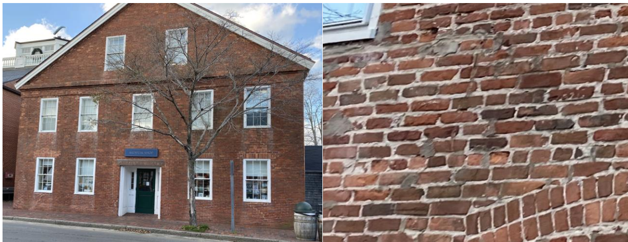
Figure 46: Possible efflorescence of bricks beneath the second story windows of the south elevation (left), and enlarged photo of cracked and spalled bricks (Right) (S. Turner).
