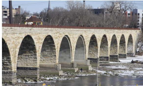
Figure 7. A drawdown being performed in the winter at St. Anthony Falls in Mississippi (Webster, 2015).
