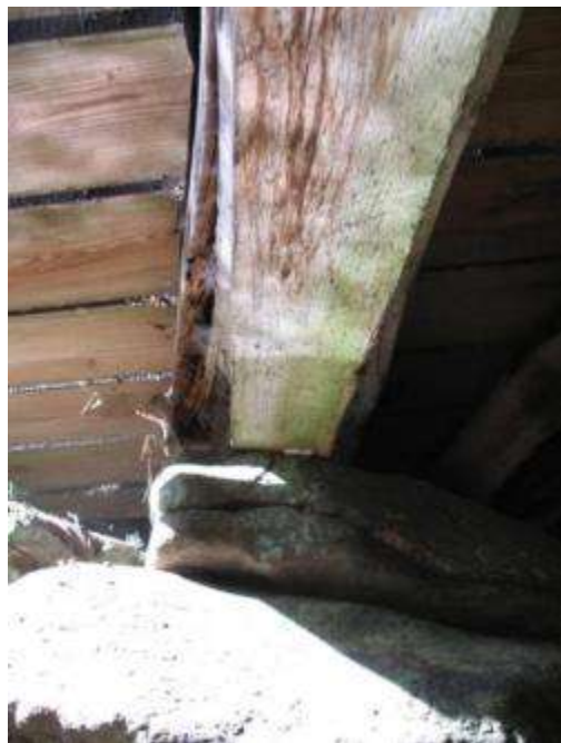
Figure 4: Failure on compression due to decay
