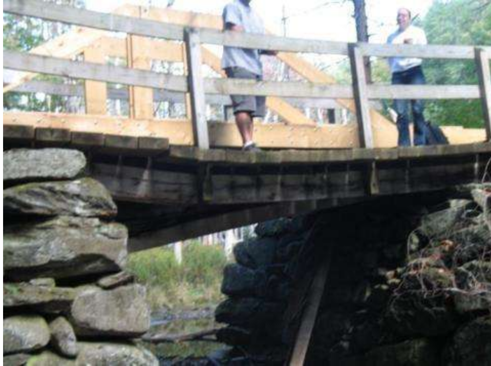
Figure 2: Excessive deflection due to overloading of remaining beams (note presence of temporary structure)
