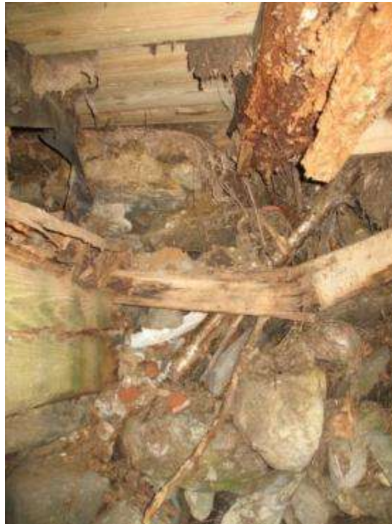
Figure 5: Decay most evident at contact with soil and water
