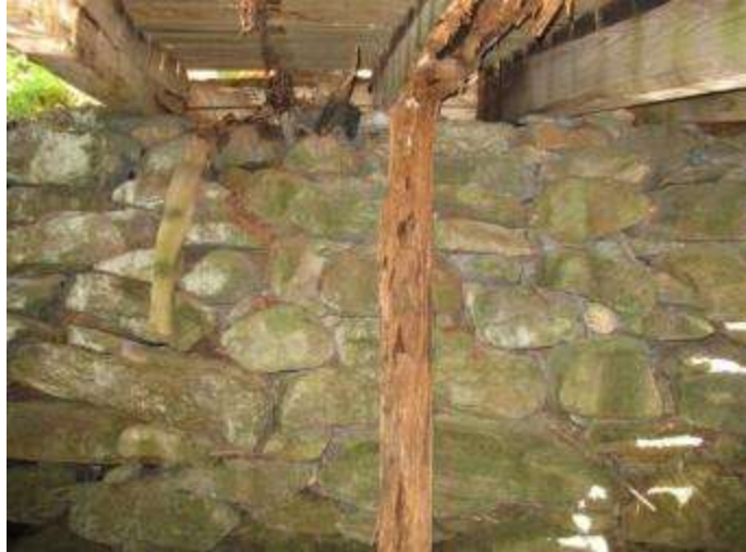
Figure 3: Rotting of entire beam length
