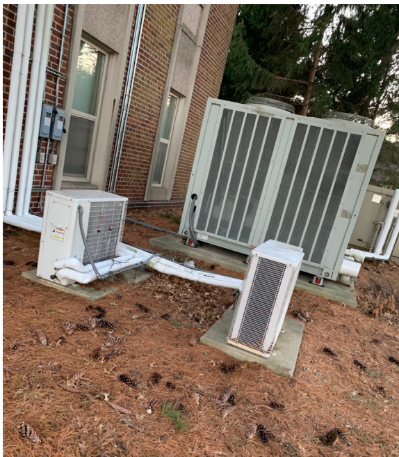
Figure 8. Photo of outdoor Condensing Units. Several different brands are installed at this location (Andrews, 2020).
