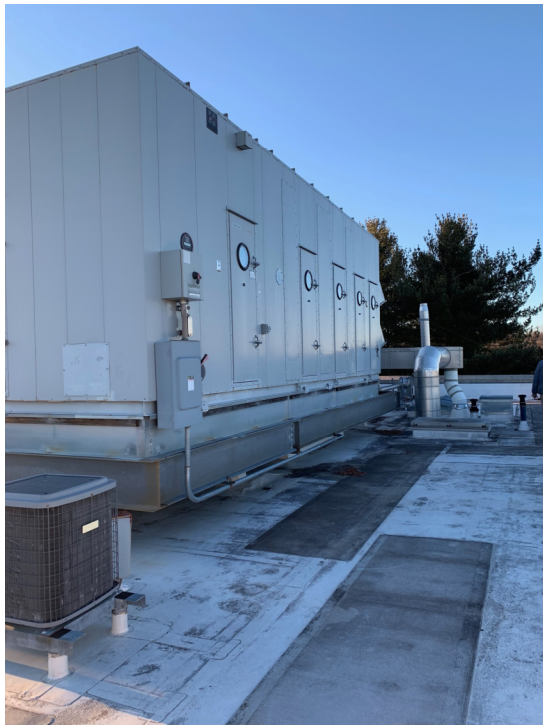
Figure 4. Roof Photo of the new combined overall exhaust system for newer half of the building. (Andrews, 2020)
