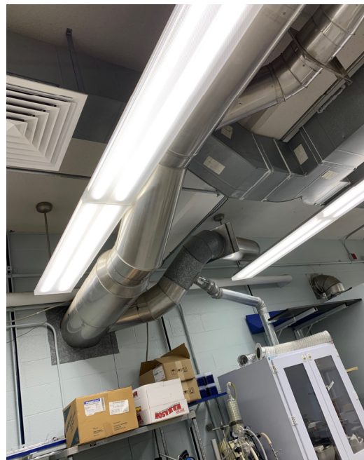
Figure 7. Photo of abandoned ducts in a second-floor research laboratory within Goddard (Andrews, 2020).
