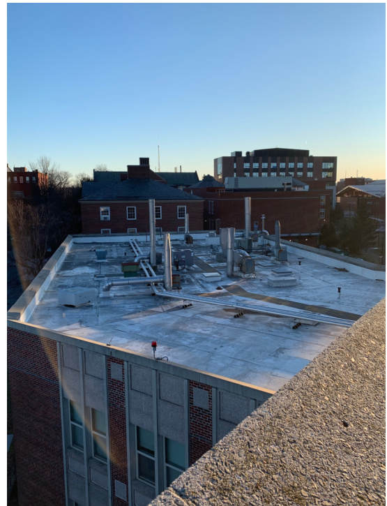
Figure 5. Roof Photo of the older, individual exhaust fans on older half of the building. (Andrews, 2020)
