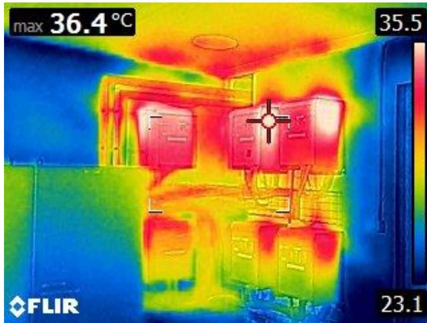
Figure 23. Substantial heat pooling due to inverter heat exhaust
