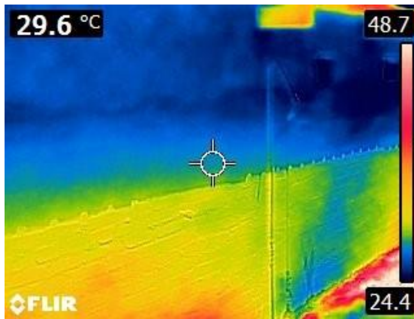
Figure 35. Depiction of the temperature gradients on the battery room external wall after being painted with heat reflective paint
