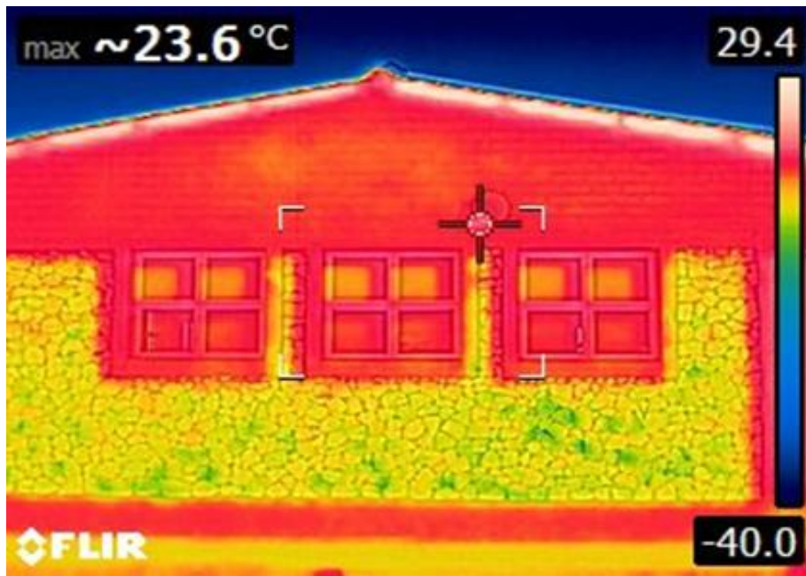
Figure 39. Community Hall temperature gradient showing how different materials affect heat gain to the building
