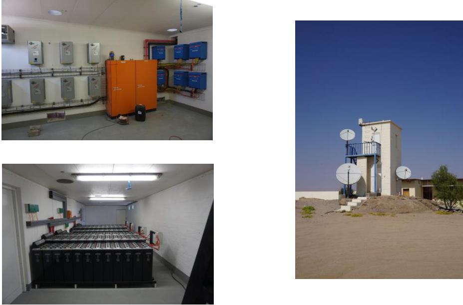
Figure 2. Photos of the Inverter Room (top left), Battery Room (bottom left), and Server Tower (right)
