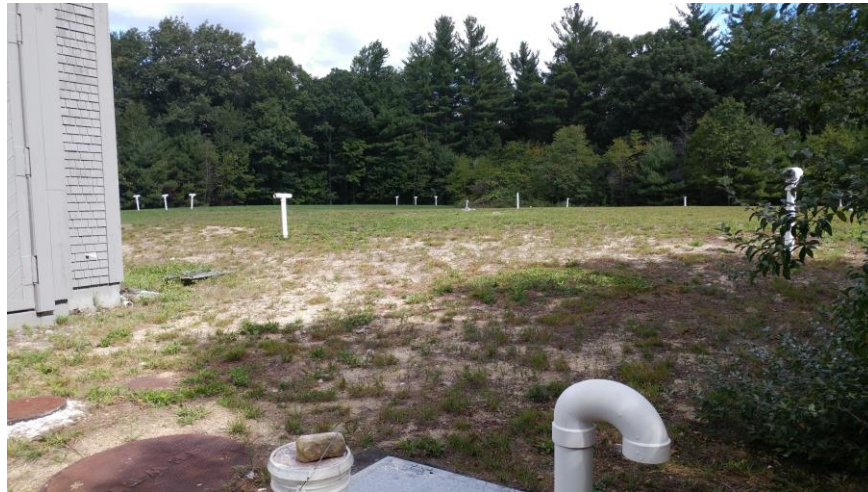
Figure 2: View of the RUCK filter system at Woodlands Village
