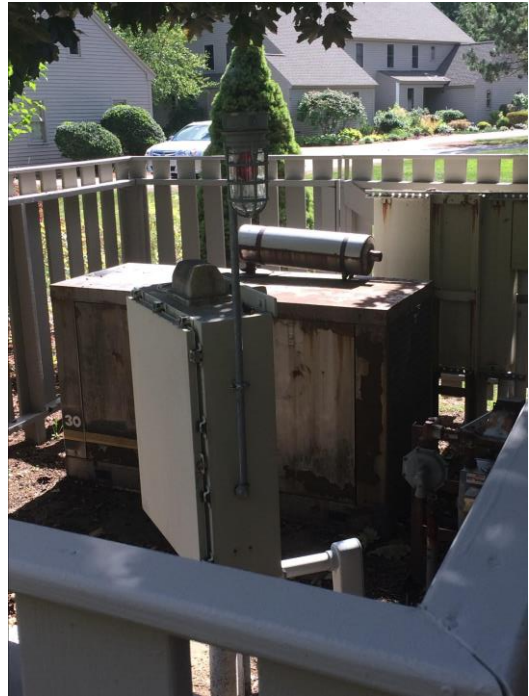
Figure 4: Main Pump Station
