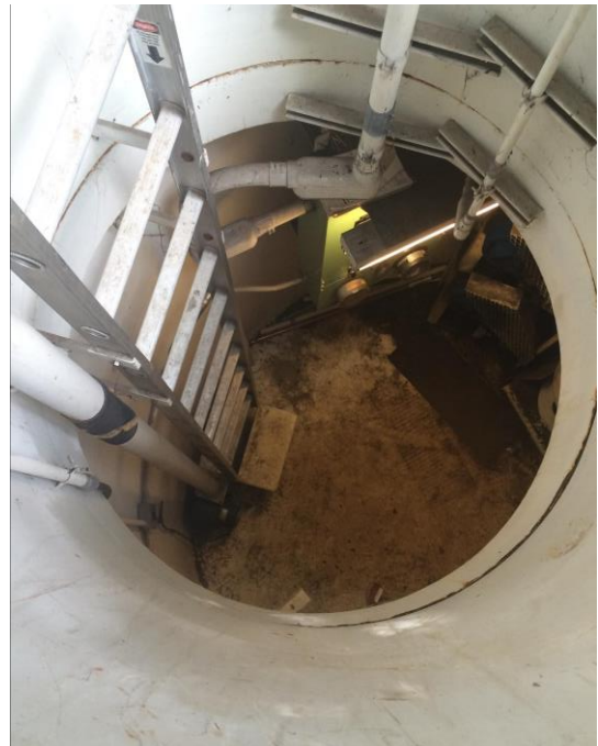
Figure 5: Pneumatic Pump Station
