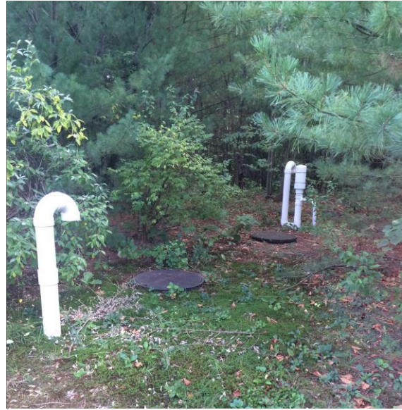
Figure 6: Septic Tank in the WWTS
