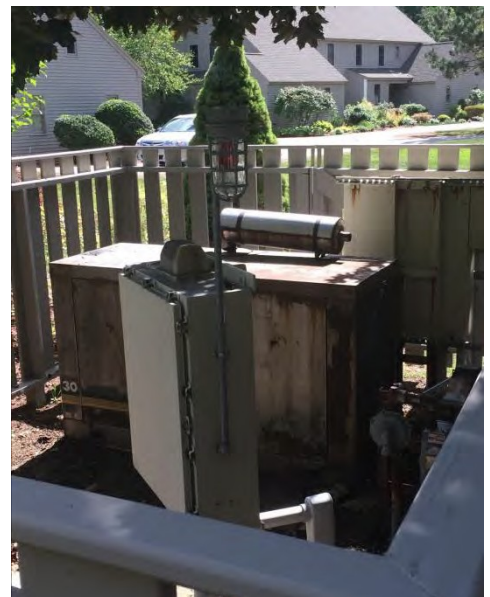
Figure 5: Main Lift Station
