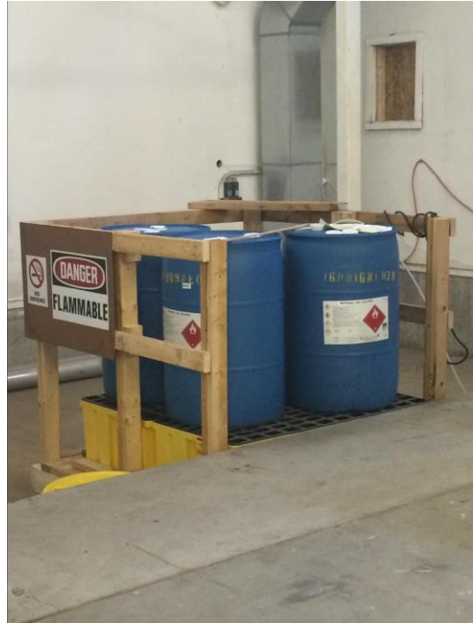
Figure 8: Methanol Barrels in the Wastewater Treatment Building
