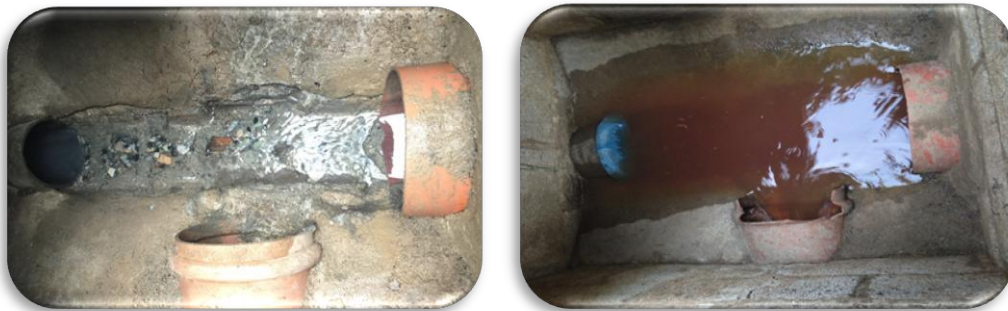
Figure 8: (left) The manhole with normal operation with dairy facility operating and (right) normal operation with dairy facility and slaughterhouse operating.
