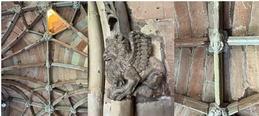
Mythological creatures in the ceilings near the Chapter House and around the cloister garden (E)
