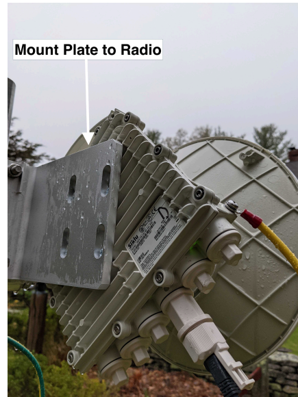
Figure 3.4: A picture of the back of the Siklu radio mounted on a non-penetrating roof mount and approximately 7 feet in the air.
