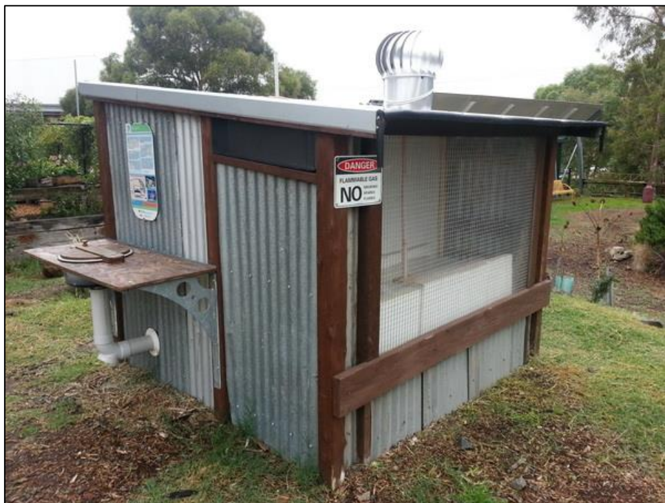
Figure 6 - Original Biogas Digester Installation and Display
