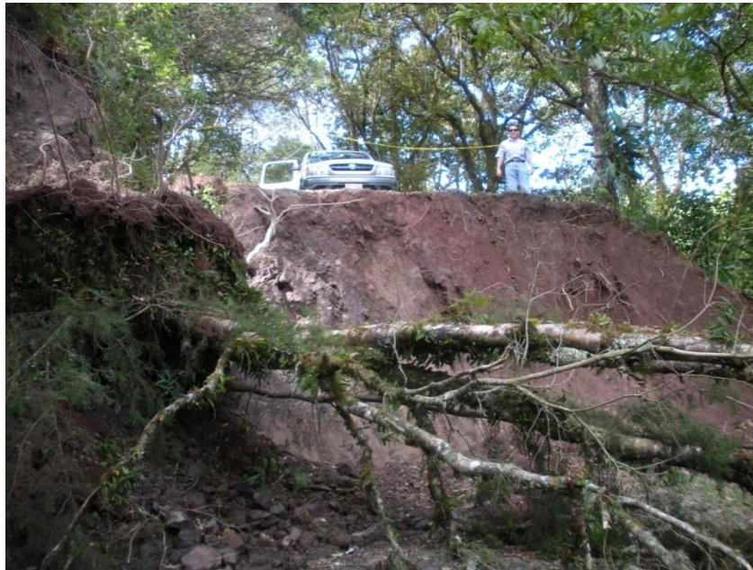
FIGURE 5: COLLAPSED ROAD IN NARANJO The road collapsed due seismic activity in the area. (Naranjo, 2008)
