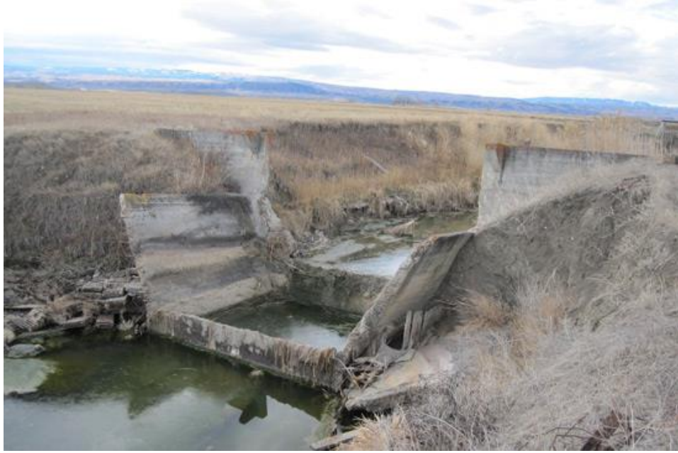
Figure 4.5: A drop weir structure system used for irrigation. (USBR, 2015)
