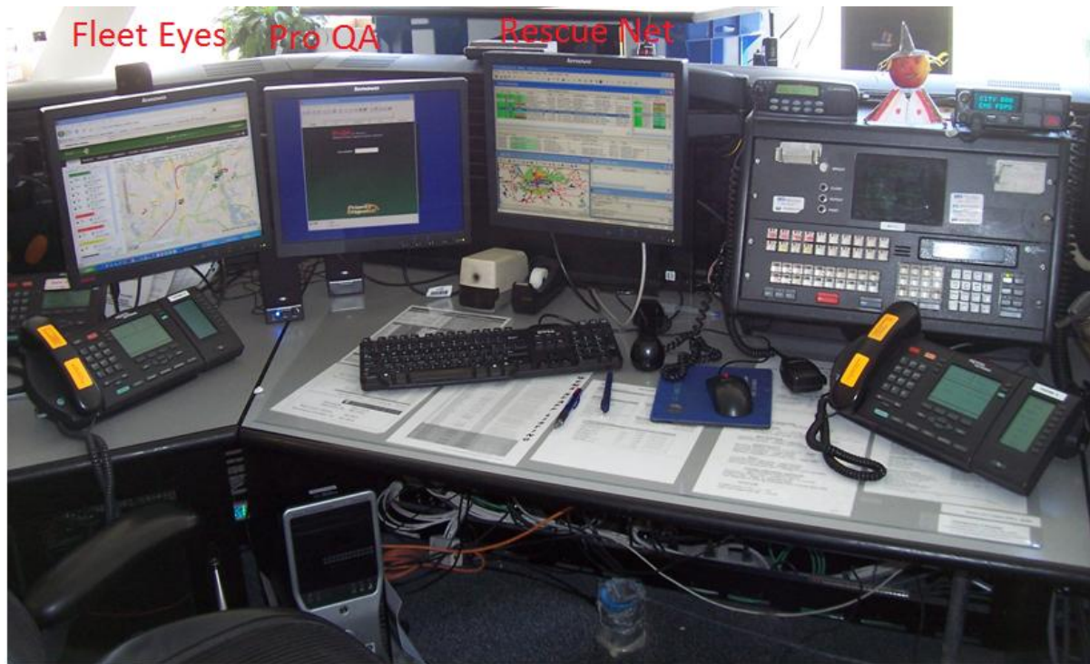
Figure 38 Dispatcher Work Station
