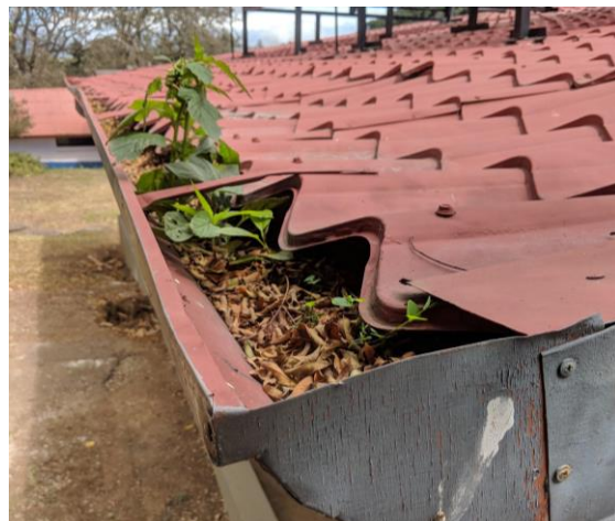
Figure 12: Example of a gutter system clogged with dirt and leaves at the Academy
