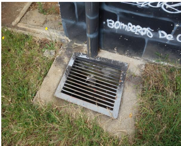
Figure 11: Example of a clogged downspout drain on the Maintenance Building
