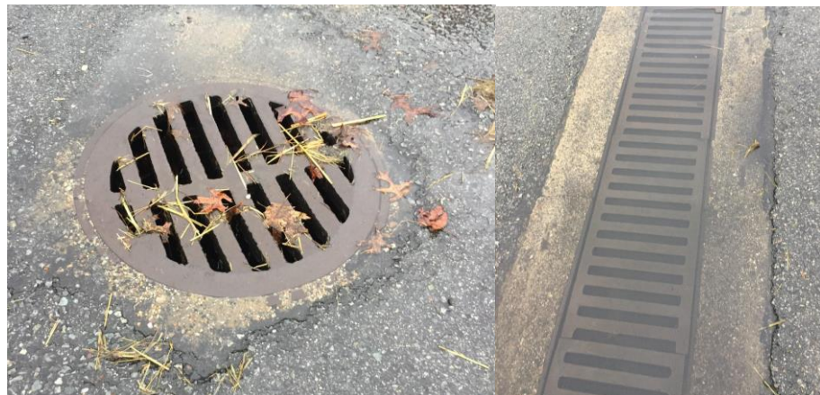
Figure B.4: Examples of drains clogged with straw and leaves used for burn material to simulate fires during training at the Massachusetts Fire Academy Scuppers on burn building clogged with straw used to simulate fire situations at the Massachusetts Fire Academy (images by Kelly Vodola)
