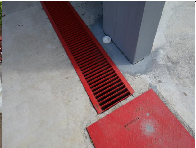
Figure A.6: Drain from wall into small tank on training pad
