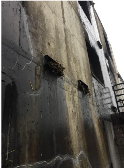
Figure B.1: Scuppers on burn building clogged with straw used to simulate fire situations at the Massachusetts Fire Academy (image by Kelly Vodola)
