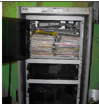
Figure E- 18: Use of server case as cabinet
