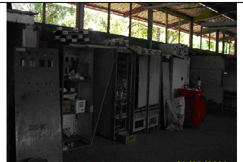
Figure E- 19: Machinery still intact
