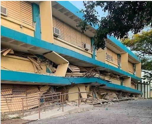
Figure 33. Building Collapsed After Earthquake. (Adapted from McPhaul, 2021)
