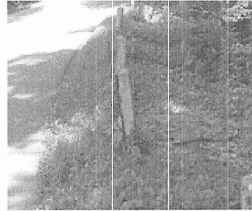
Figure 10 Poor Guard Rail
