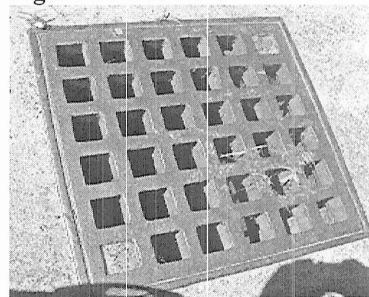
Figure 19 Excellent Storm Drain
