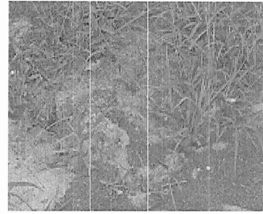
Figure 16 Poor Storm Drain
