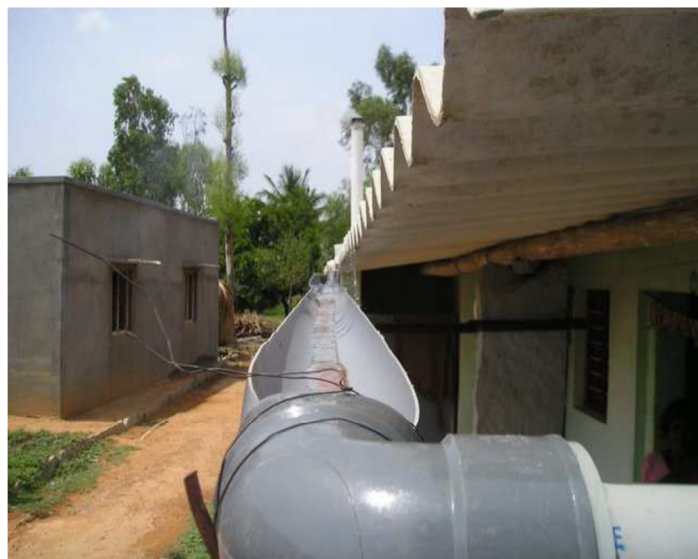
Figure 14 – Clean PVC gutter to catch rainwater
