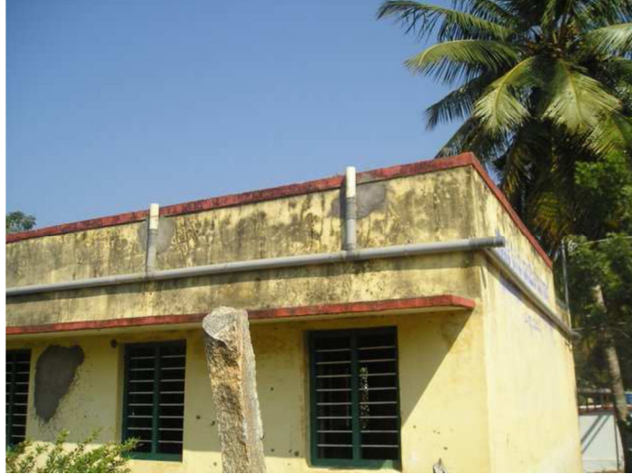
Figure 15 – Gutter systems installed in a school in Karnataka
