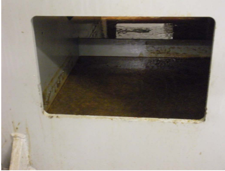
Figure 8: Contaminants in coolant sump
