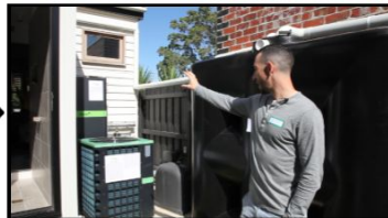
"The engine room of our sustainable home..." "Our Heat Pump and Storage Tank..."
