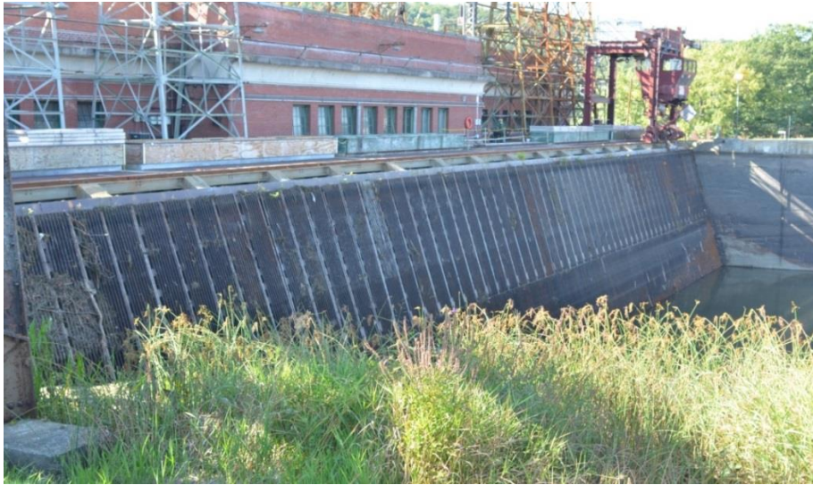
Figure 3 - Bar rack orientation at Cabot Station, Turners Falls (Photo Credit: Steve Amaral, 2012).
