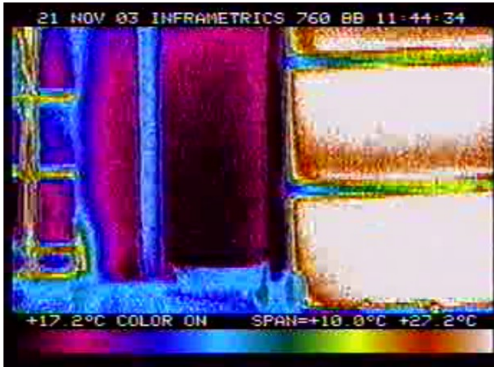
Figure 16a. Thermal Image of Second Floor New Window and Adjacent Old Window
