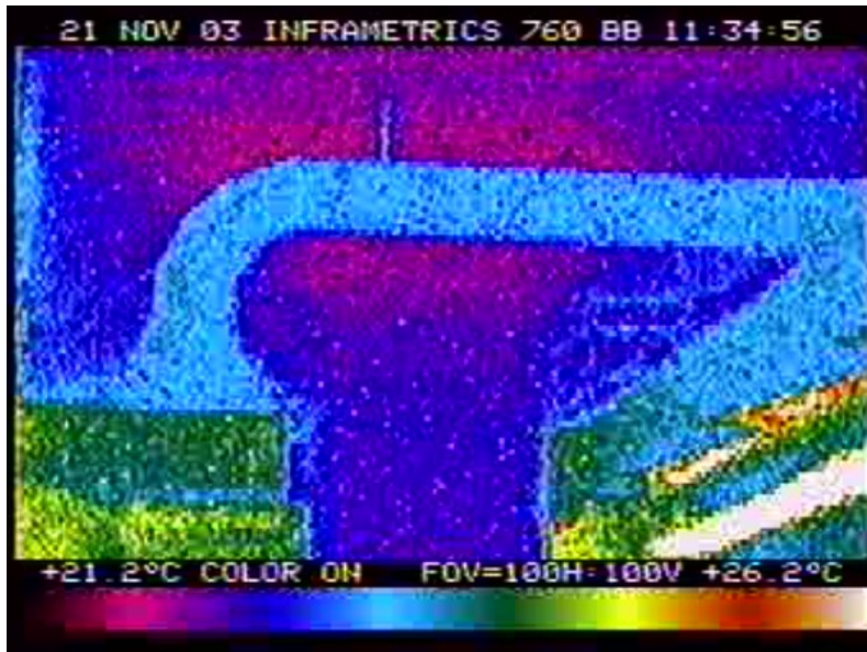
Figure 15a. Thermal Image of Ductwork in Davis Publications
