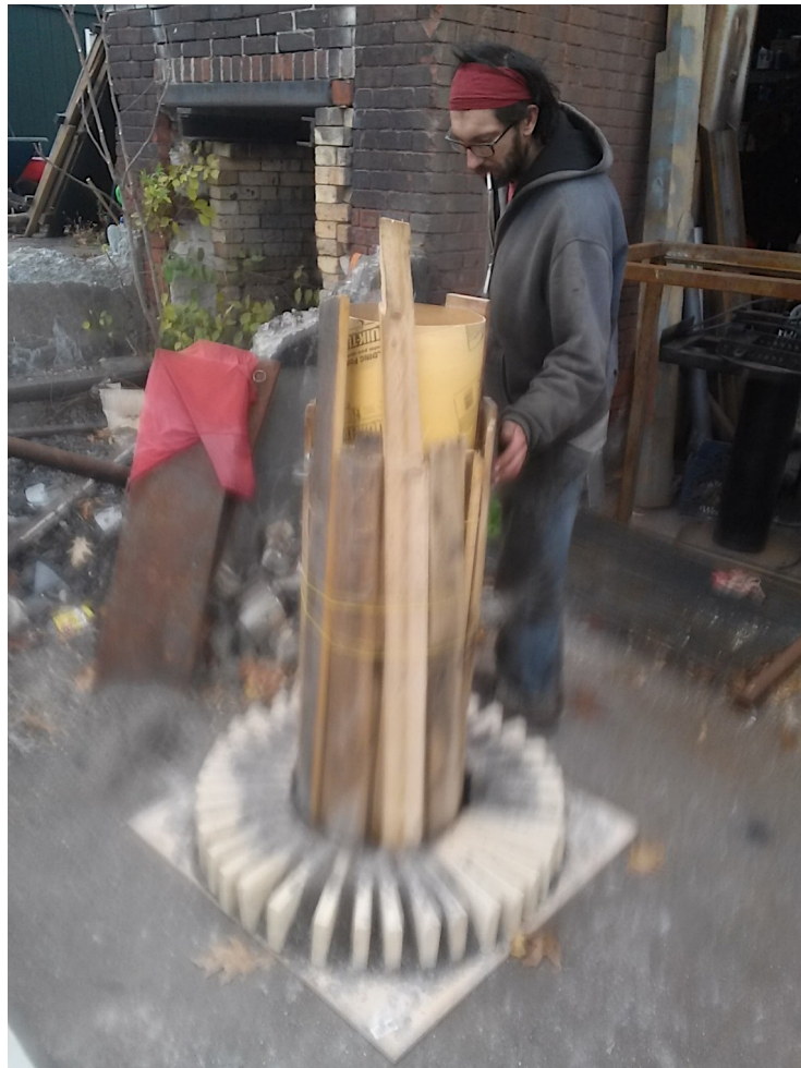
FIGURE 38. FURNACE STRUCTURAL SUPPORT TUBES.
