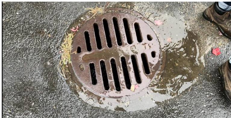
Figure 5: Storm drain at the EcoTarium
