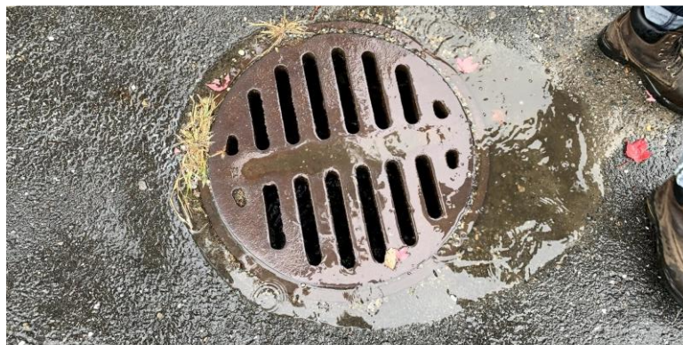
Figure 5: Storm drain at the EcoTarium
