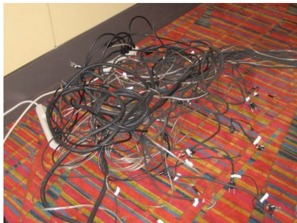
Photo 11: Troubleshooting can be a Mess
