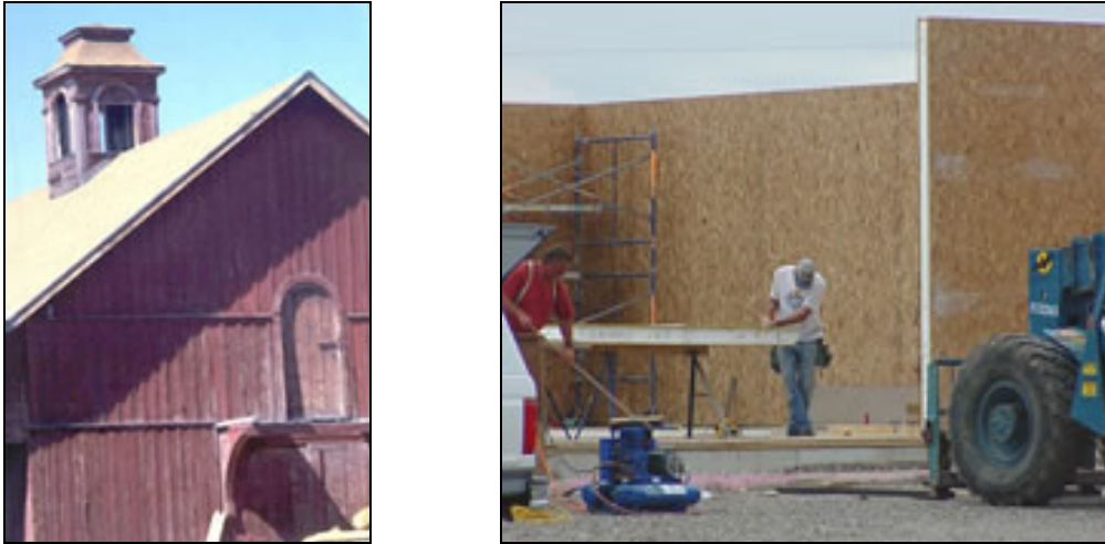
Figure 2: Barn Cupola (left) and Barn construction using insulated materials (right) Source: http://www.attra.org/attra-pub/agbuildings.html
