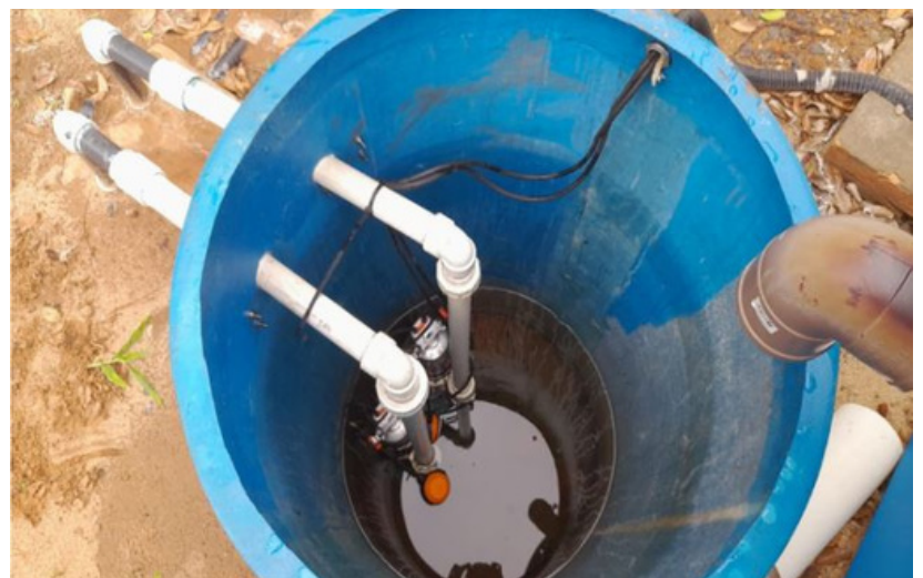
Figure 5: The two pumps that move the treated water to the aljibe (cistern).
