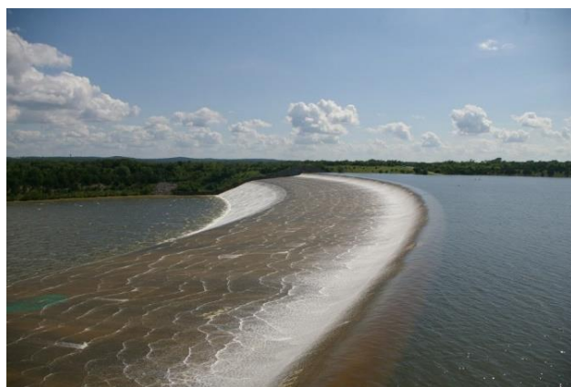
Figure 4. An Emergency Spillway Being Used in Texas. Note. From Spillway, Wikimedia Commons
