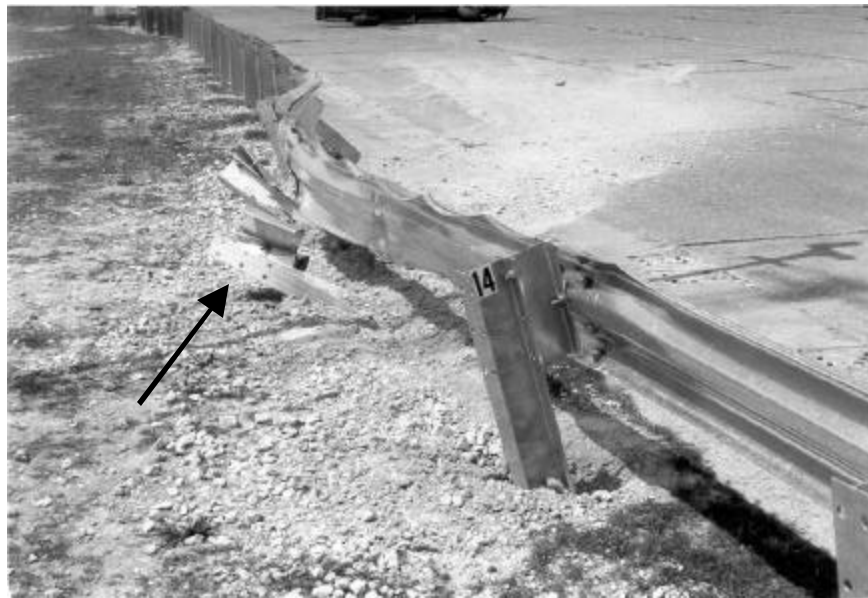
Figure 19. Deformation of a steel W150x13.5 post showing a lateral torsional buckling failure. (6)
