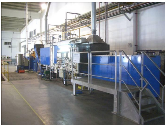
Figure 4 Mesh Belt Furnace
