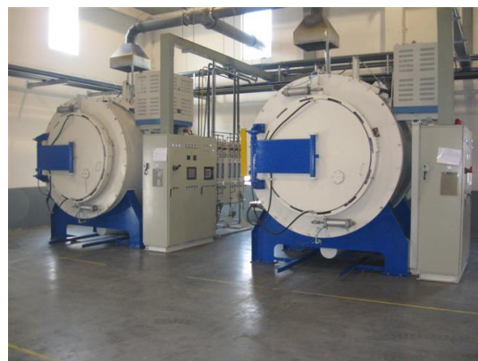
Figure 3 Vacuum Nitriding Furnace
