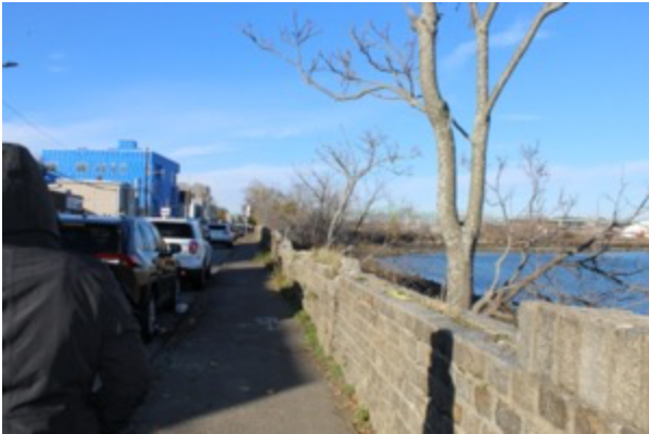
Figure 34. Erosion at Base of Wall
