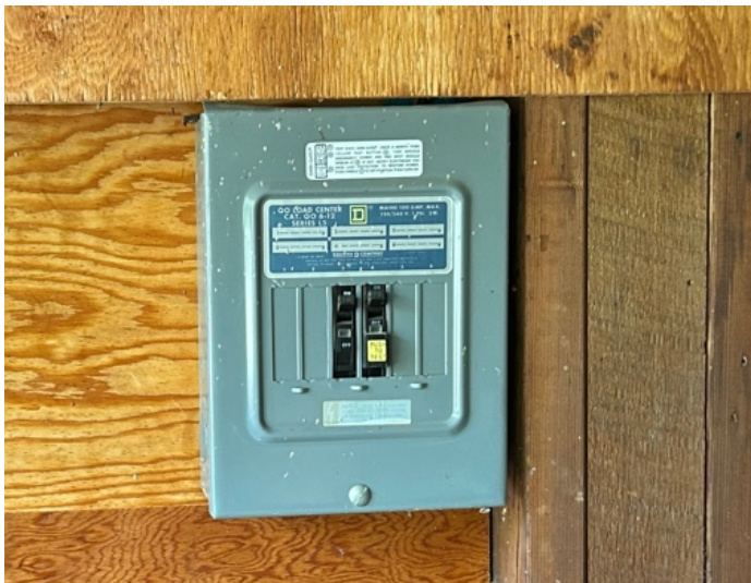
Figure 7: Current Breaker in the Red Bike garage
