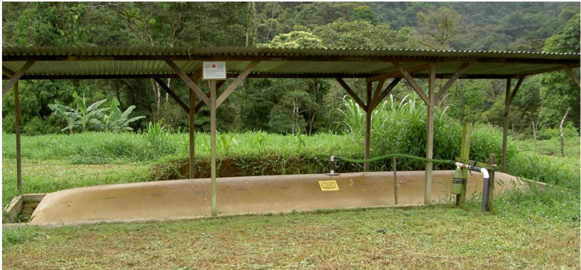
Figure 6: Solano Farm Polyethylene Anaerobic Digester
