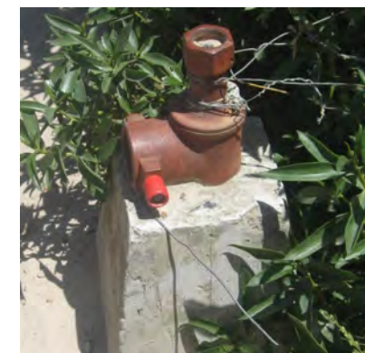
Fire Hydrant in C Section
