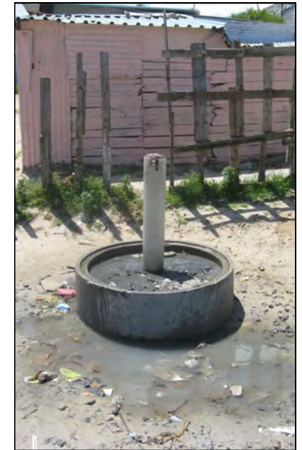
Standing Water Due to Overflow
