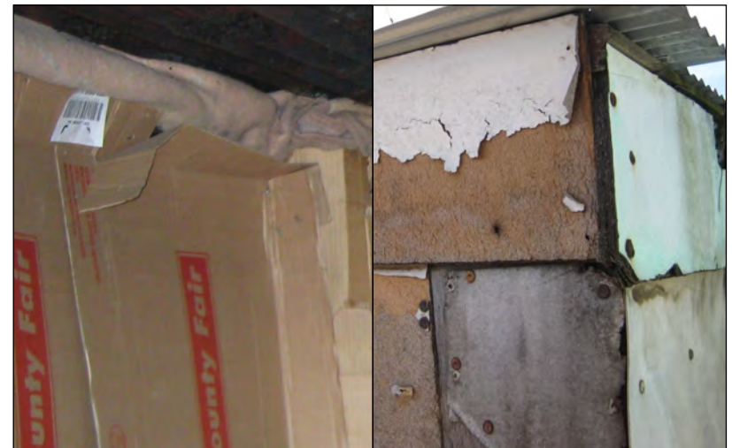
Figure 5-8: Current shack insulation methods include cardboard on walls, newspaper and other random materials in gaps and boards on the exterior.
