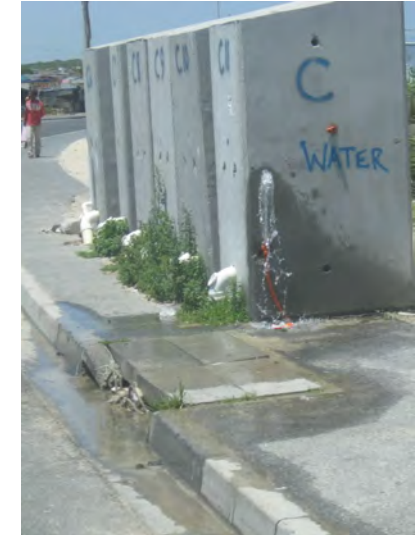
Water waste and associated problems are common throughout South Africa as evidenced by this leaking toilet in a settlement outside of Khayelitsha
