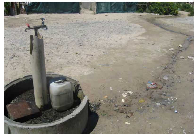
Even on the taps in arguably better condition, issues with leakage and waste are still prevalent and troublesome
