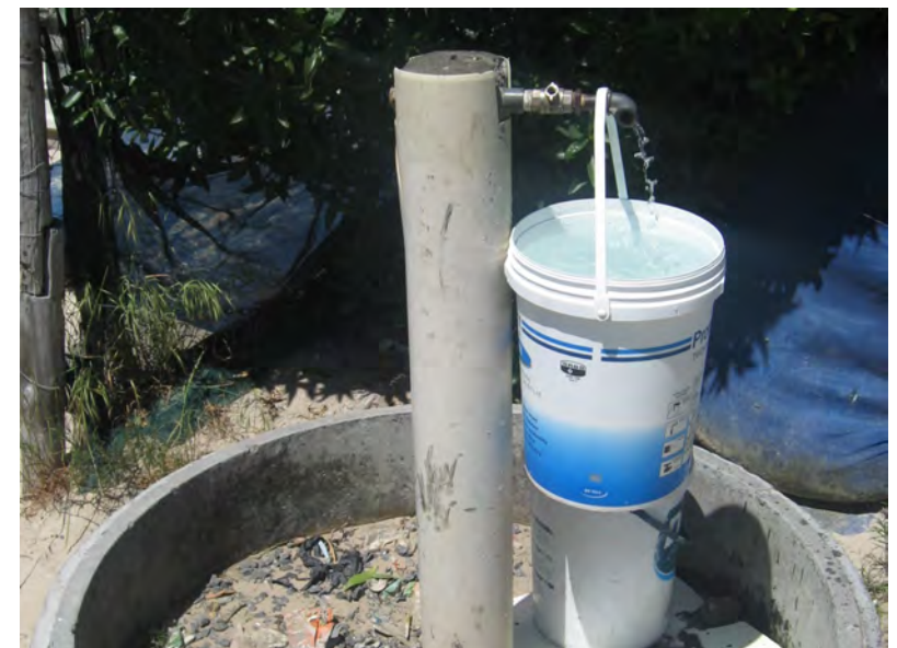
Buckets are commonly hung on piping for easier access
