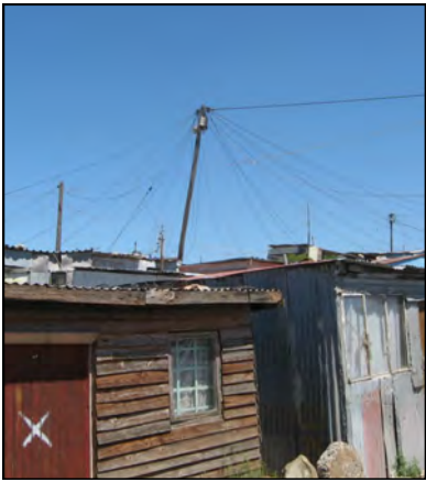
Figure 4-3: Official connections fan out from power poles to boxes.
