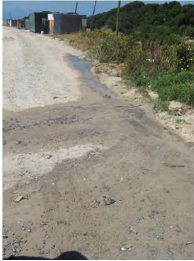
Wasted water flowing down a street causing erosion and creating stagnant pools.
