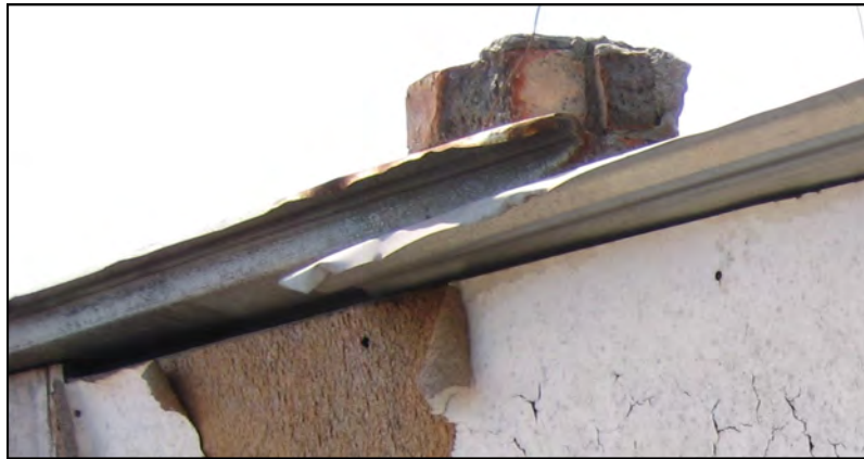
Figure 5-7: Typical shack roof which often leaks during the wet, winter season.
