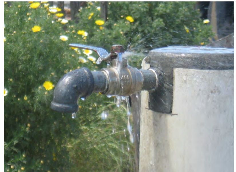
The conditions of faucets deteriorate over time and with prolonged usage tend to leak and break without regular maintenance.
