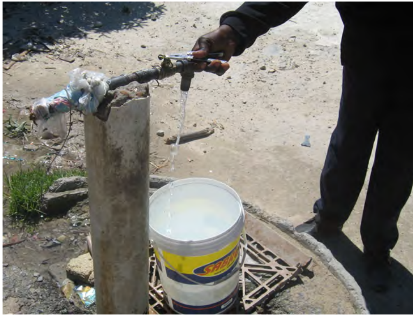
An example of a tap with a broken pipe and a missing handle. Residents have to use pliers or a makeshift wire device when handles go missing
