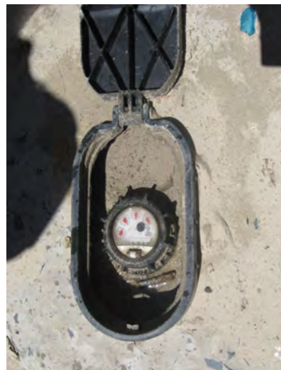
Individual tap water meters are buried next to each tap. Gauges are seldom checked and tap usage is generally unknown
