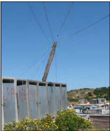
Figure 5-4: Those with informal connections must put up their own wires and poles.
