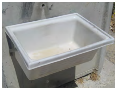
An existing (but broken) sink available for washing on the side of a pour/flush group
