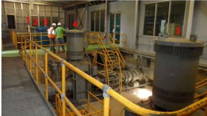
Figure 10 - The Five Vertical Pumps at the Paraíso Pumping Station (Photo taken by Cindy Lin, 2012)
