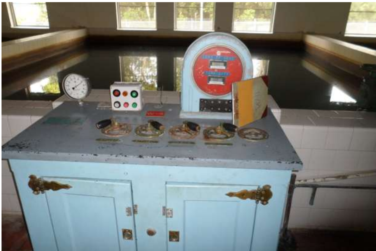
Figure 14 - Sedimentation Basin at the Miraflores Filter Plant (Photo taken by Shelby Miller, 2012)
