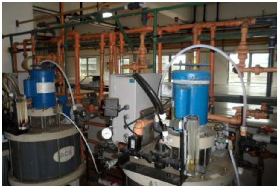
Figure 12 - Chemical Additives at the Miraflores Potable Water Plant (Photo taken by Cindy Lin, 2012)
