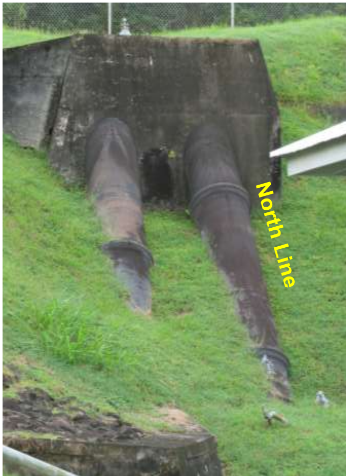
Figure 8 - Two 30 Inch Pipelines Leaving Paraíso Pumping Station (Photo taken by Cindy Lin, 2012)
