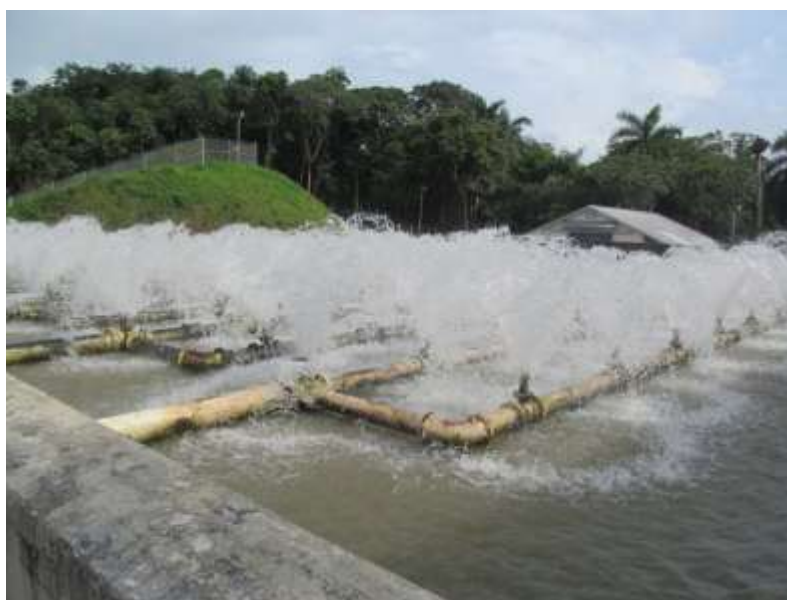
Figure 11 – Water Aeration Process at the Miraflores Filter Plant (Photo taken by Shelby Miller, 2012)
