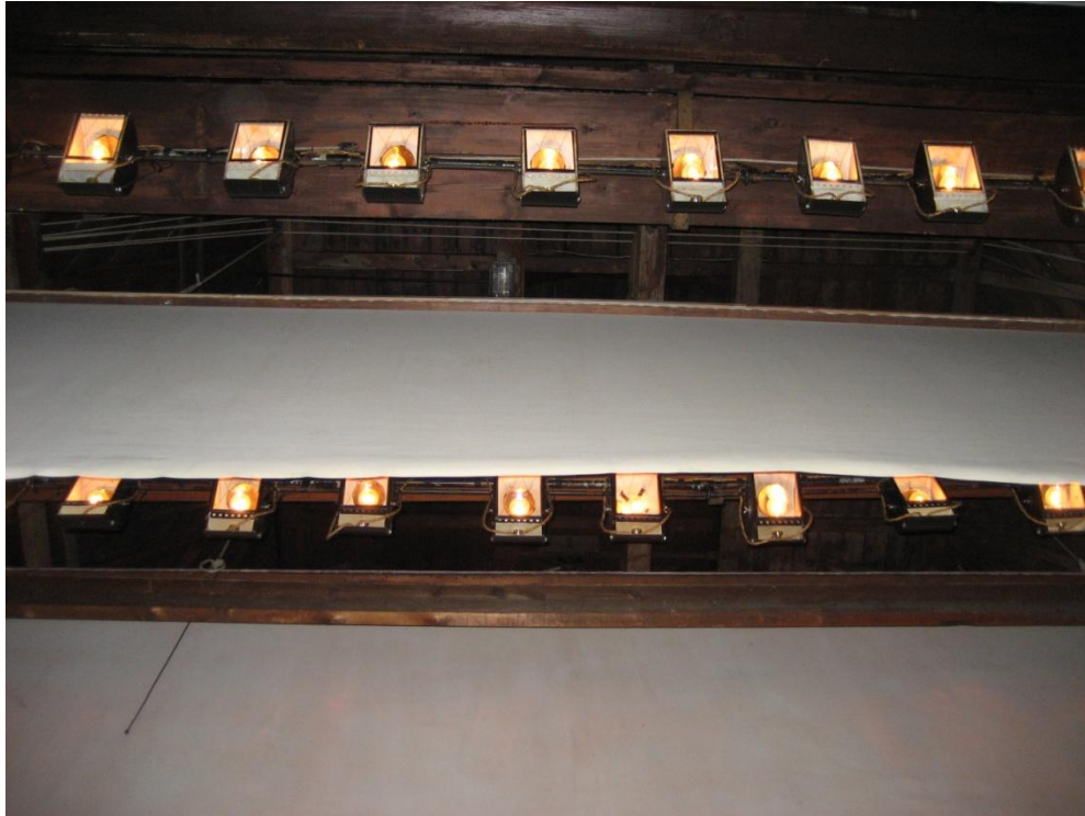
Figure b.1.10 Electric lights present in the Nornansfield Theatre.
