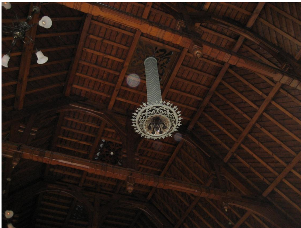
Figure b.1.11 The original main gas house light fixture in the theatre.
