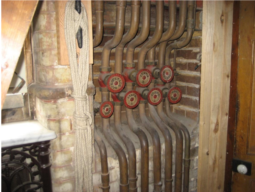
Figure b.1.14 The original gas pipes that were part of the gas lighting system at the theatre.
