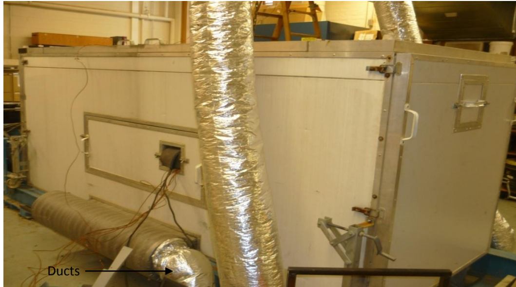
Figure 14: Hot Air duct under environmental chamber
