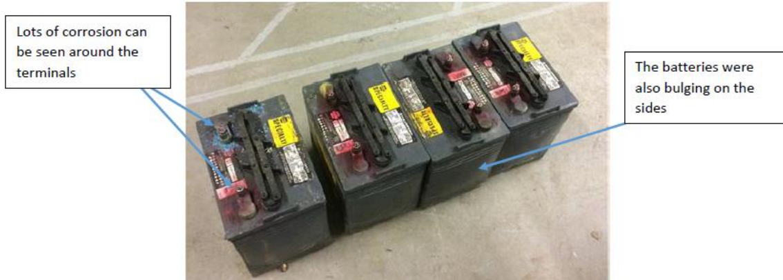
Figure 5: State of the Batteries in 2016 [9]
