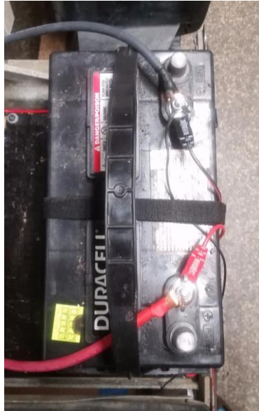
Figure 20: Close Up of Mounted Series Battery
