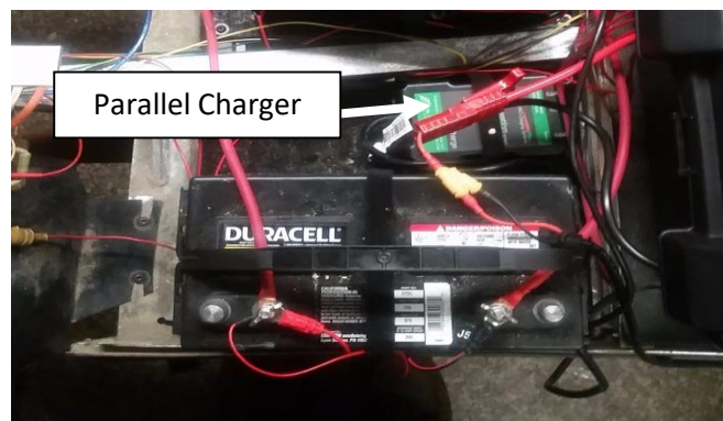
Figure 23: Parallel Battery Charger Mounted
