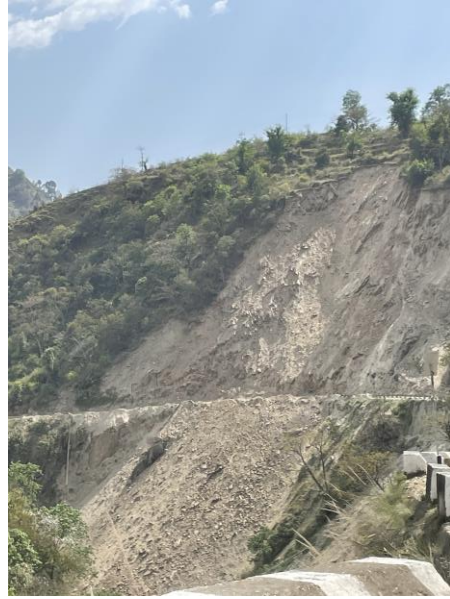
Figure 14: Example of dramatic landslide that had disrupted road traffic just outside IIT Mandi's campus in Kamand (Photo credit: Fox, 2023).
