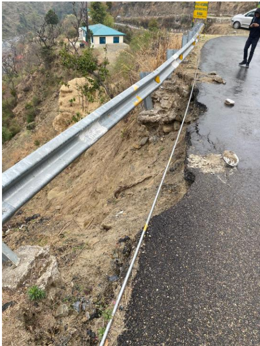
Figure 15: Erosion causing a landslide on a local mountain road making it dangerous for drivers (Photo credit: McGonigle, 2023).
