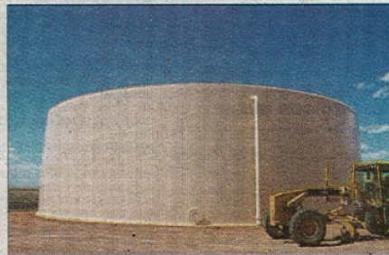
Las Campanas has built a 2-million-gallon tank to hold treated effluent at the Santa Fe wastewater-treatment plant. The water is then pumped seven miles to irrigate the luxury development's golf courses, which use 450,000 to 800,000 gallons a day.
