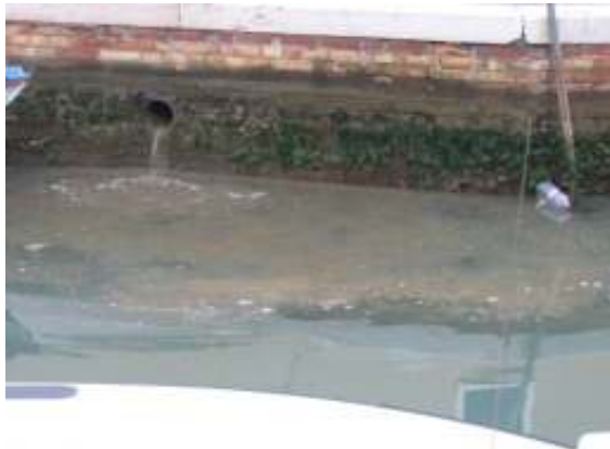
Figure 7: Raw sewage flowing out of piping and directly into the canal
