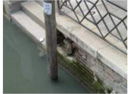
Figure 15: Damage in canals, including the restoration of docks is maintained simultaneously
