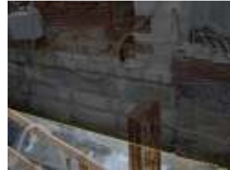
Figure 14: The bottom layer of construction, highlighted in yellow shows the concrete that is used to reinforce the wall
