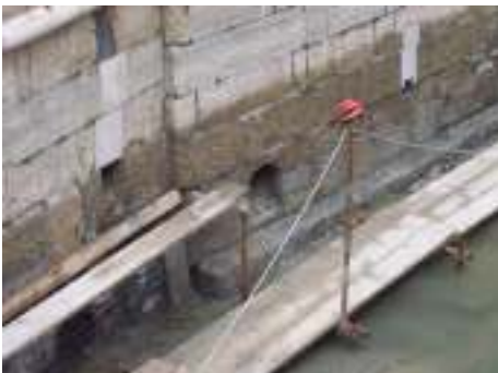
Figure 11: Usually hidden beneath the surface of the water, sbocchi can be seen when canals are drained for maintenance. The sbocchi allow sewage to flow from the collettori into the canals.
