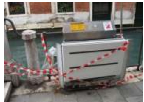
Figure 23 – One of the Servoscala systems that is out of order
