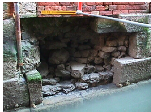
Figure 20: Example of a hole in a canal wall
