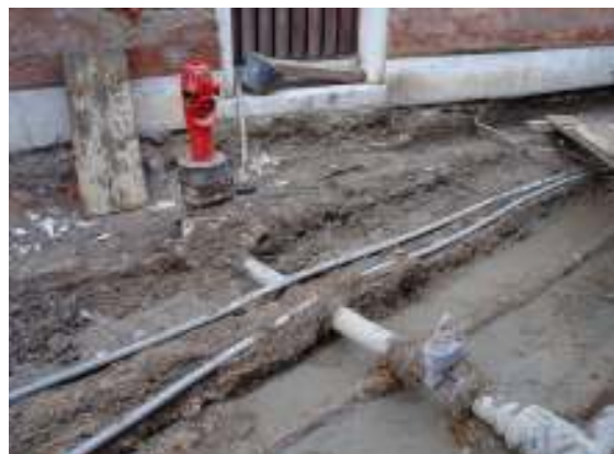
Figure 2: A section of the various utilities exposed for maintenance work. The new fire fighting network is still being installed within the city. Implementation began after the old fire fighting methods were
