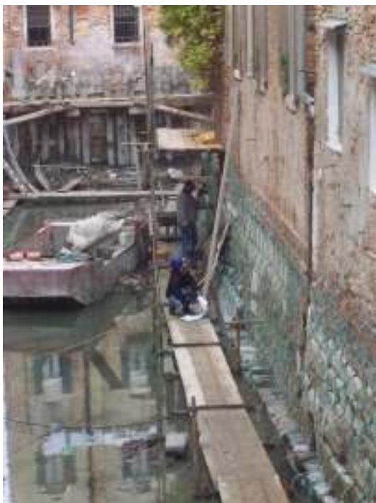
Figure 32: This shows the technique used to fill mortar during the restoration of canal wall linings
