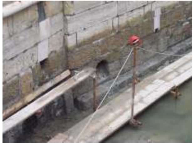
Figure 22: After a canal is dredged and drained, sewer holes are able to be cleared out
