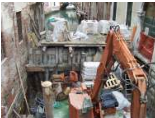
Figure 30: Machinery, including the grab-bucket used to scoop out and remove sediment away to designated treatment sites.
