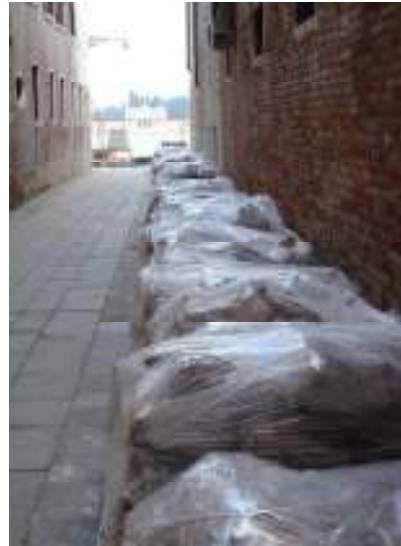
Figure 12: Pallets of paving stones being stored while work is performed on the near by fondamente.
