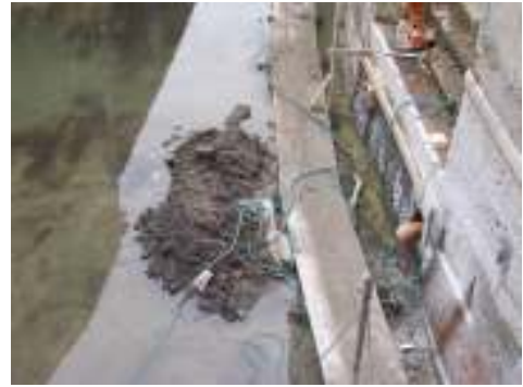
Figure 31: Accumulation of sediment at the bottom of the canal
