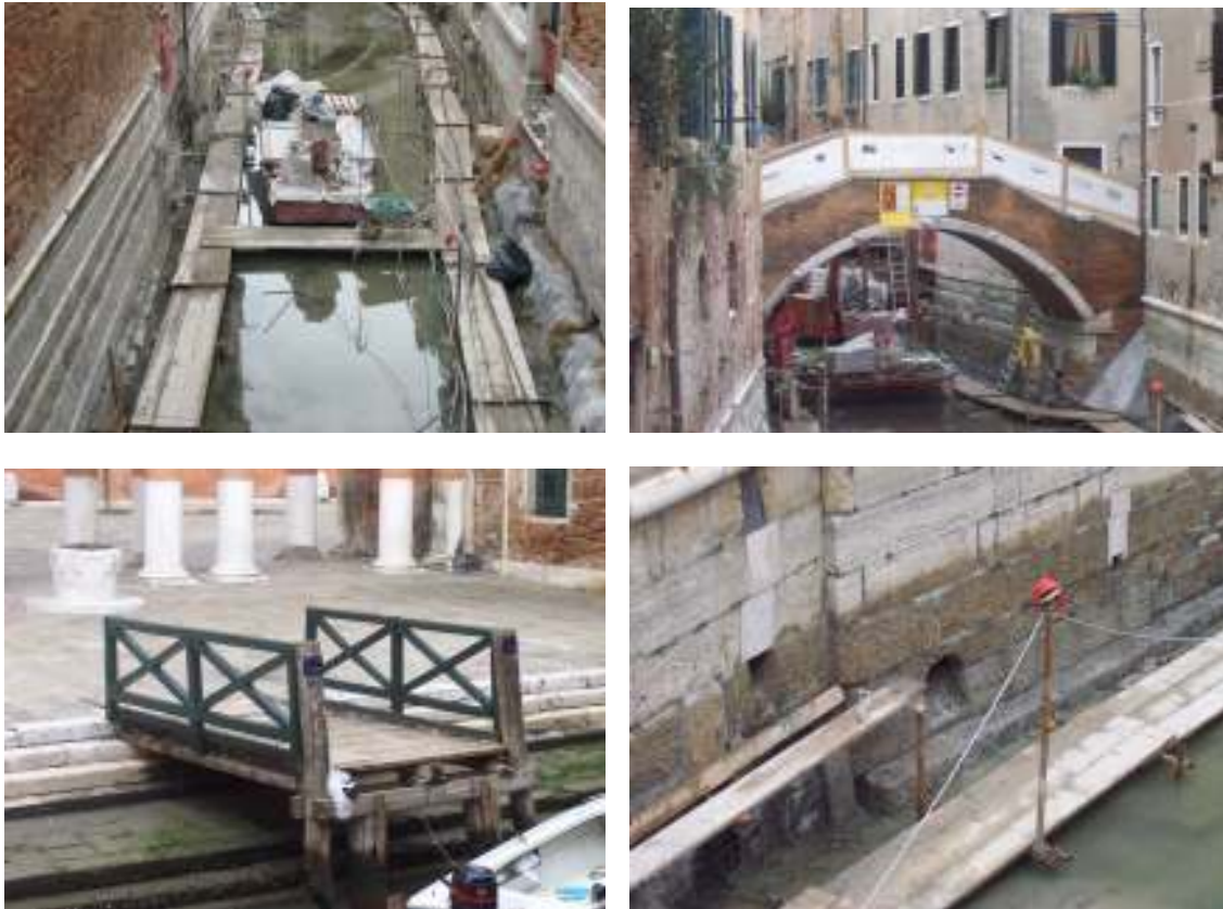
Figure 1 (top, left): This is a drained canal during the dredging stages of canal maintenance. The linings of canal walls are also restored during this process. Maintenance generally takes about six months to complete. Insula is currently in the third and final phase of their canal maintenance plan. Figure 2 (top, right): Bridges are maintained following the canal maintenance schedule. The undersides of bridges are repaired by Insula, the leader in urban maintenance. Insula has currently repaired over 200 bridges of the 473 bridges in the city of Venice. Figure 3 (bottom, left): Wooden over structures are built over stone docks throughout the city that are difficult to use according to tide levels. This is a method boaters and cargo transporters use to adapt to the unusable conditions of 32% of the 1300 docks in Venice. Figure 4 (bottom, right): Sewer pipes drain directly into the canals causing sewage to accumulate at the bottom of the canal. The holes, which are under the waterline are maintained while the canal is empty. Currently the city is discussing the implementation of a new vacuum sewer system in the historical area.
