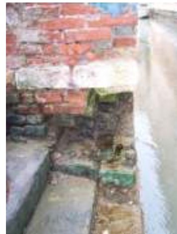
Figure 23: A damaged canal wall in need of serious maintenance
