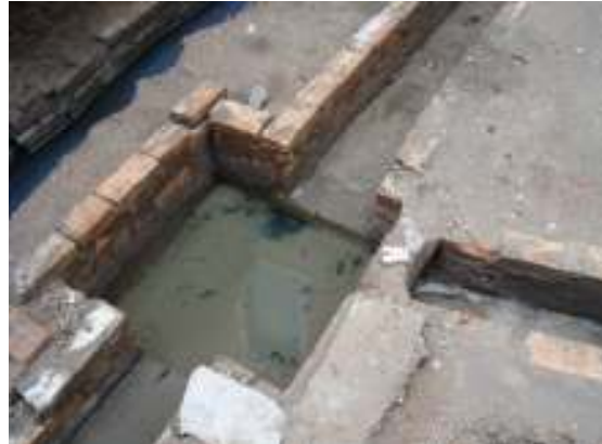
Figure 10: A portion of the collettori exposed for maintenance work. Underground, multiple collettori merge into one major channel that ultimately carries the waste to the canal.
