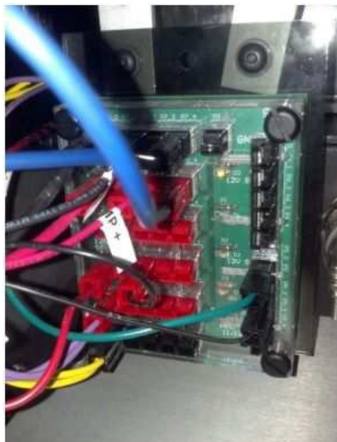
Figure 6V: Power distribution board
